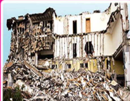
STRUCTURAL COLLAPSE (Building collapse)
